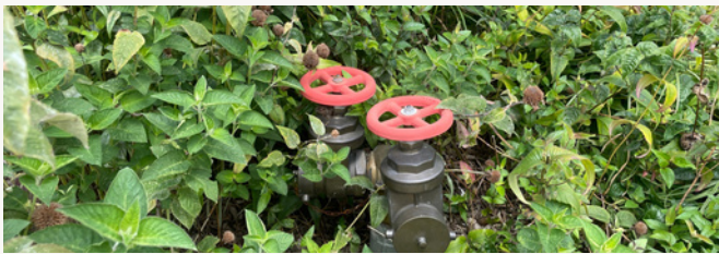
11.) Continue towards The Glade to discover the standpipes for the firefighters
